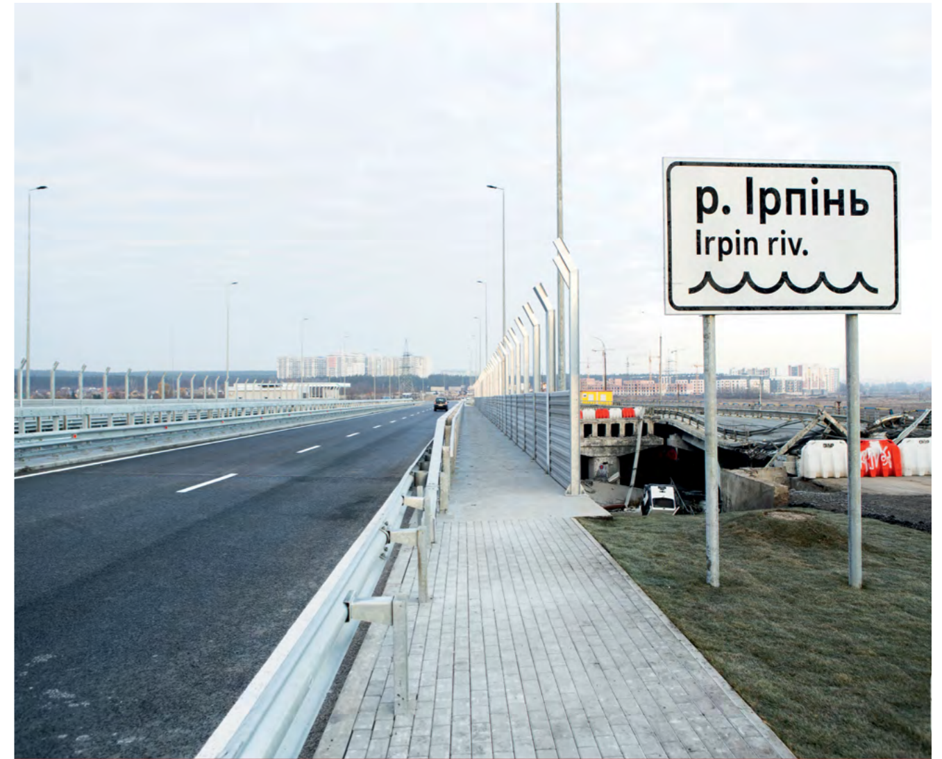
Repairing wartime damage in Ukraine: Onur Group completed reconstruction work on Irpin Bridge north of Kyiv in November 2023. The bridge had been partially destroyed during the Battle of Kyiv in the first weeks of the invasion in spring 2022. Onur Group has been involved in a number of reconstruction projects and road repair works in different regions of Ukraine following liberation from Russian occupation.
